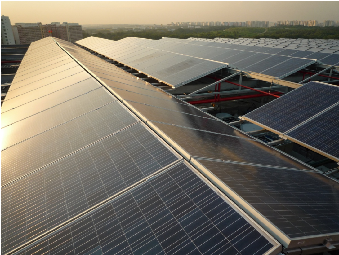
Caption: Phoenix Solar is a market leader in commercial and industrial photovoltaic rooftops in Singapore. This PV system was installed atop the Tampines Mall in the East of Singapore.
