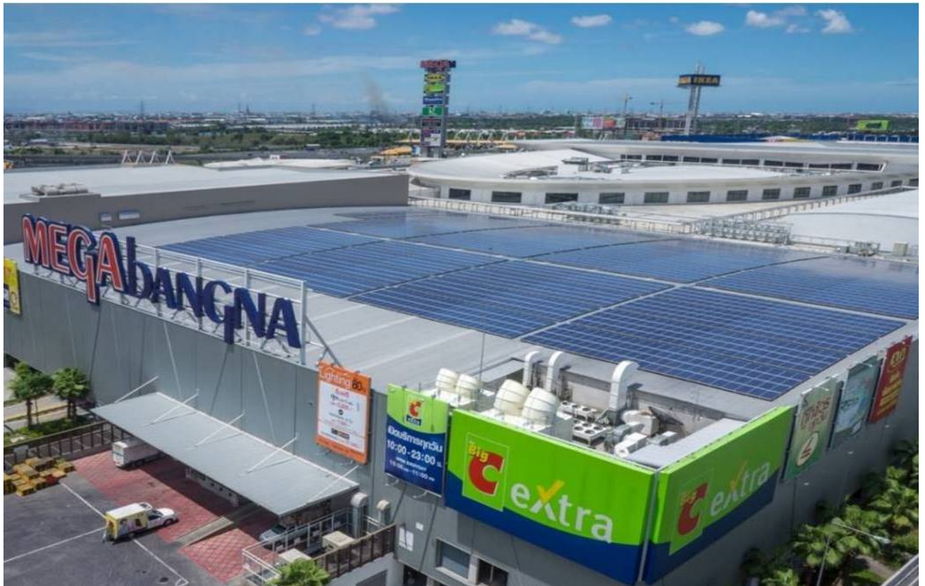
Caption: Phoenix Solar engineered 1 MWp photovoltaic system atop IKEA Southeast Asia's Megabangna mall in Thailand.
