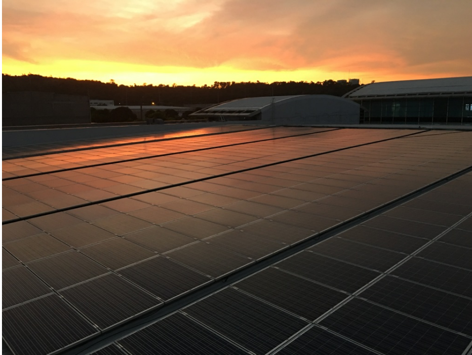
Caption: Sunrise on the Philippines. The first photovoltaic system designed and built by Phoenix Solar Philippines atop the Continental Temic Electronics facility near Manila.
